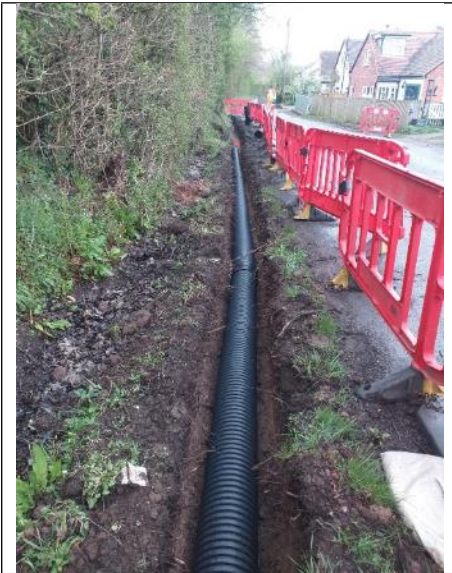
Figure 8: Part of the new drainage system to tackle a flood issue in chapel Lane, Bransford. (Annex A, Table A1, item C14 refers.)
