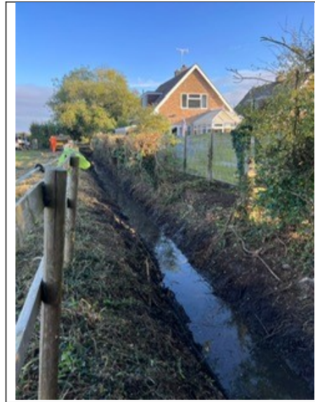
Figure 9: New ditching to reduce flood risk to highway and property, Babylon Lane, Bishampton. (Annex A, Table A1, item C13 refers.)
