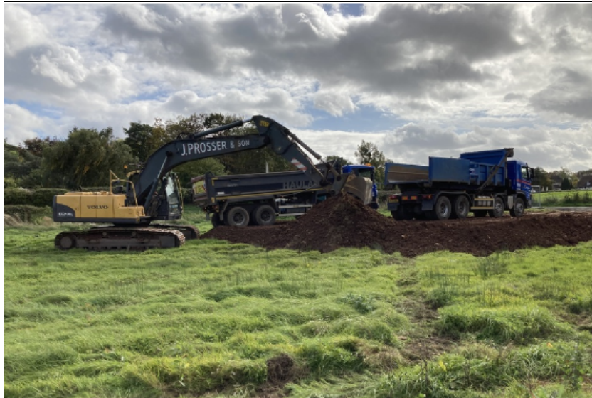
Figure 13: Soil being transported to Severn Stoke for use in the flood alleviation scheme. (Annex A, Table A2, item P7 refers.)
